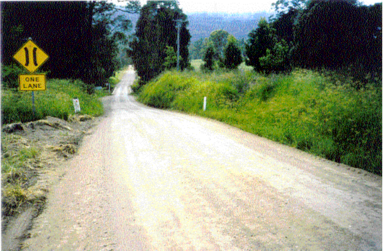
Photo 11 Renolith - cement treated sandy clay soil / gravel pavement section of Wonglepong Road after 7 days.
