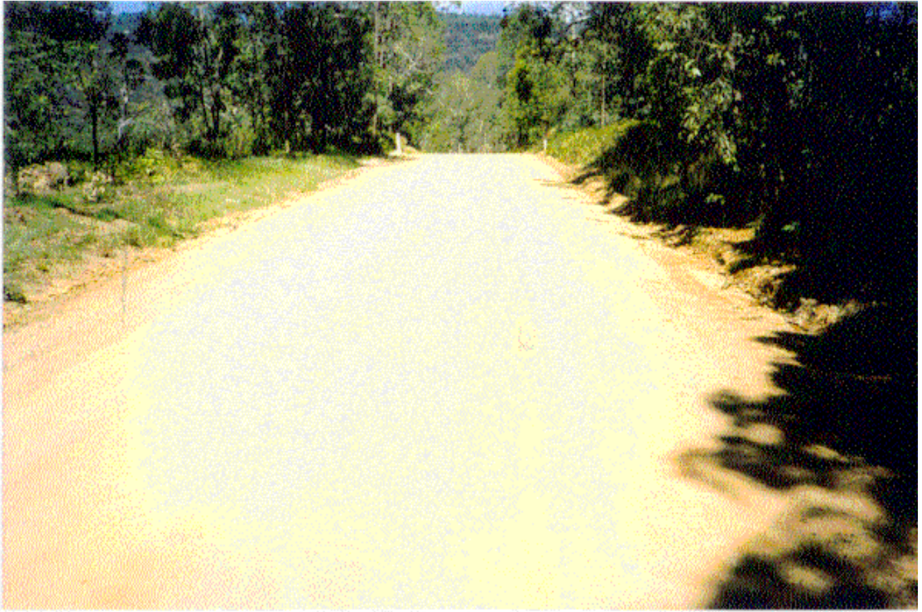
Photo 17 Renolith - cement treated orange sandy clay pavement section of Wonglepong Road after 28 days.
