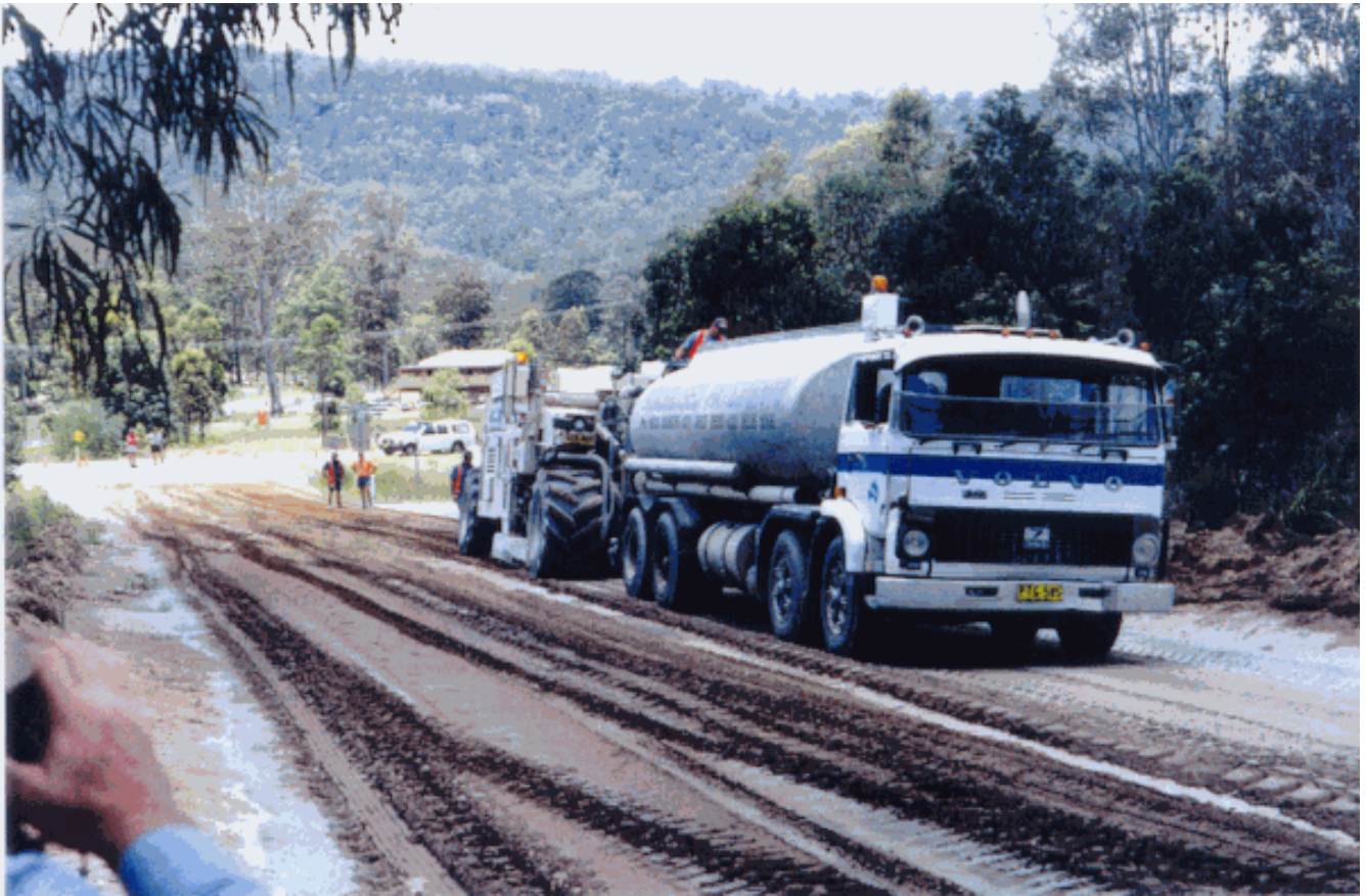
Photo 4 Final mix of pavement by Reclaimer mixer unit direct fed by water truck prior to compaction.
