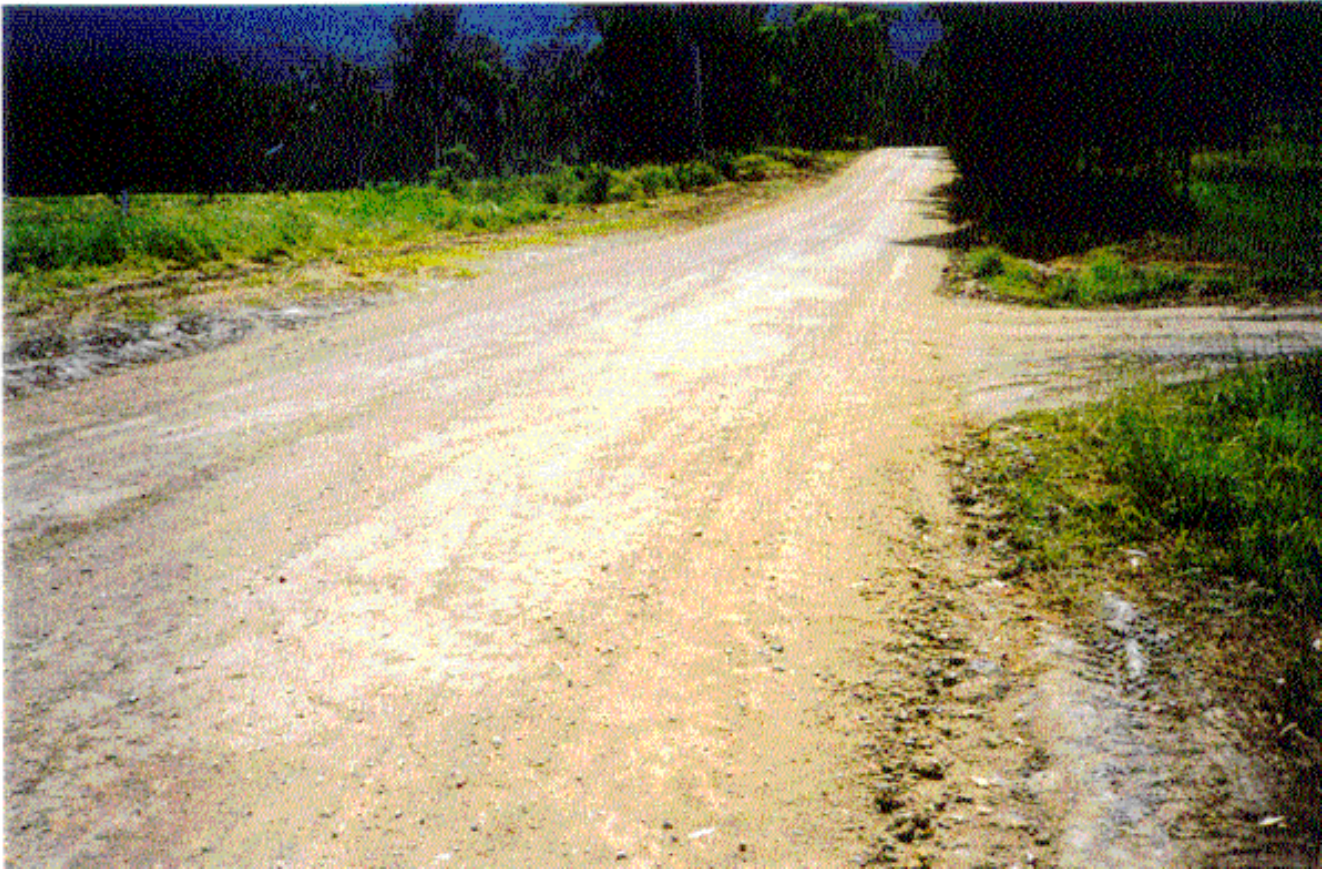
Photo 9 Renolith - cement treated black soil pavement section of Wonglepong Road after 7 days.
