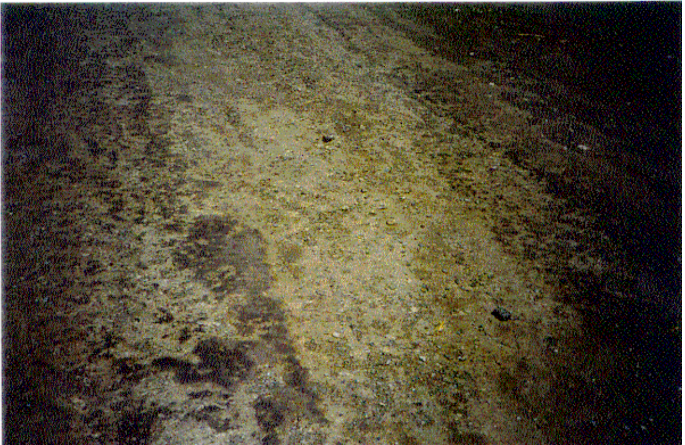
Photo 20 Renolith - cement treated black soil pavement material at bridge approach after 28 days.
