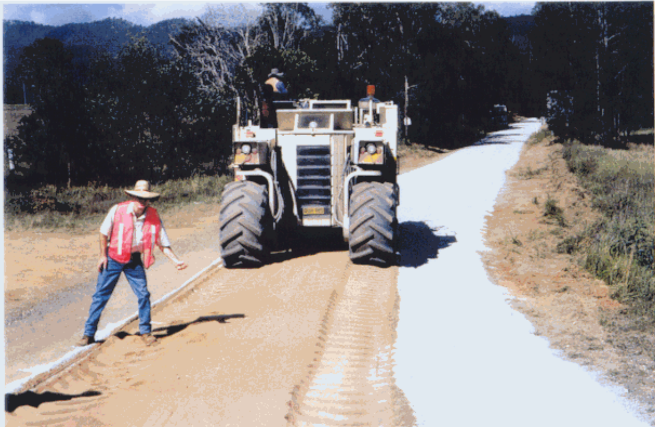
Photo 2 CMI RS-650 Reclaimer mixer unit mixing cement and pavement material to a 200mm depth.
