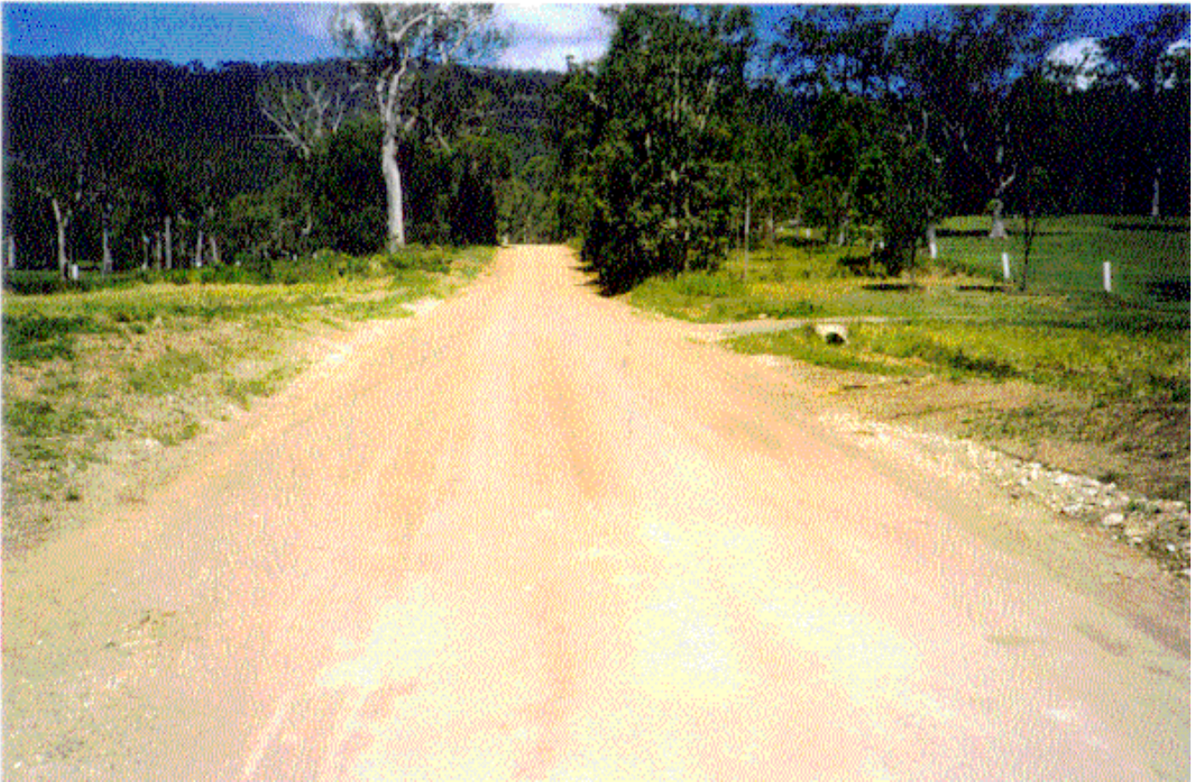
Photo 19 Renolith - cement treated black soil pavement section of Wonglepong Road after 28 days.
