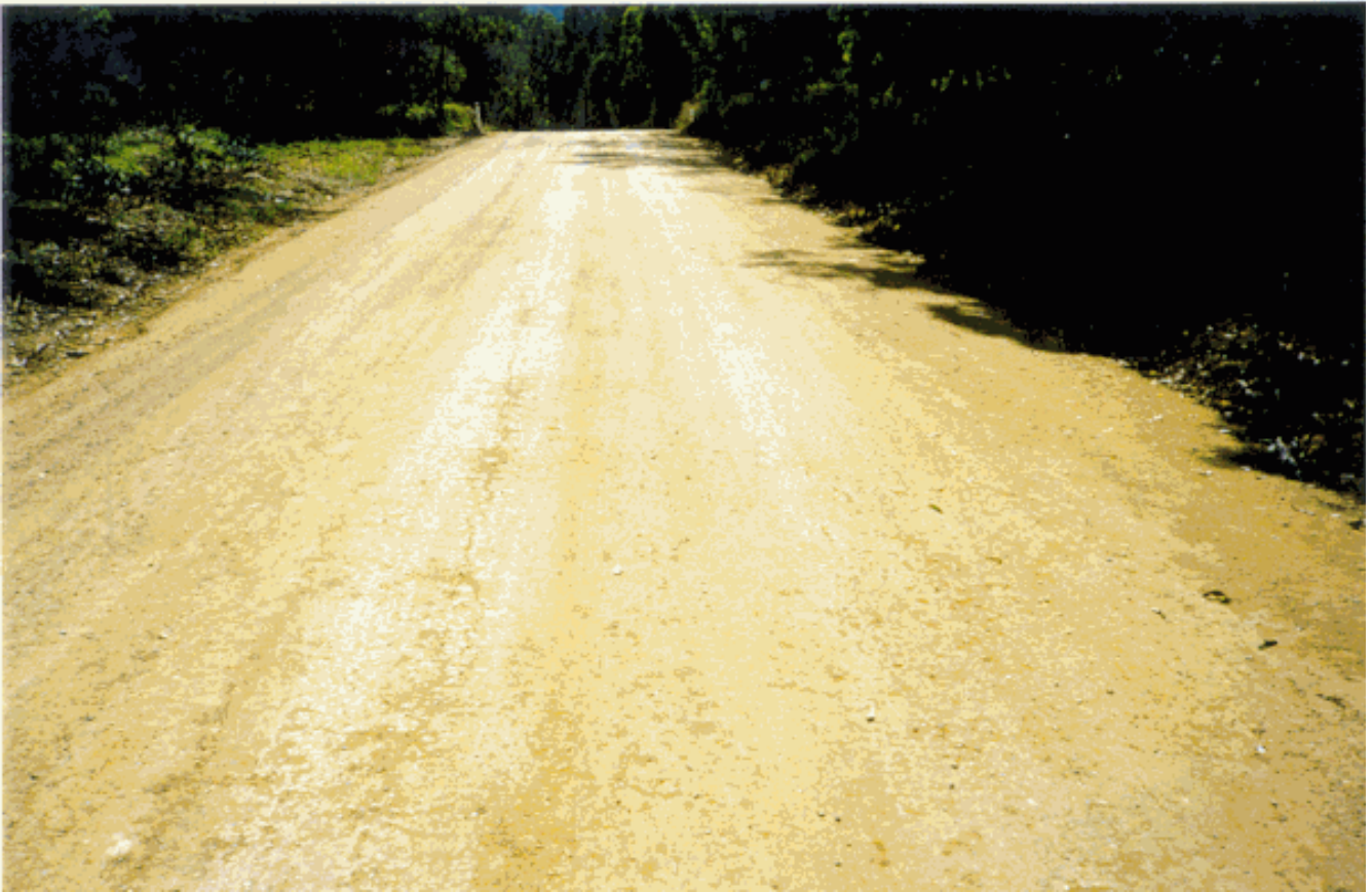
Photo 7 Renolith - cement treated orange sandy clay pavement section of Wonglepong Road after 7 days.
